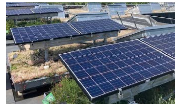
Innovation with solar panels and green roofs for biodiversity
