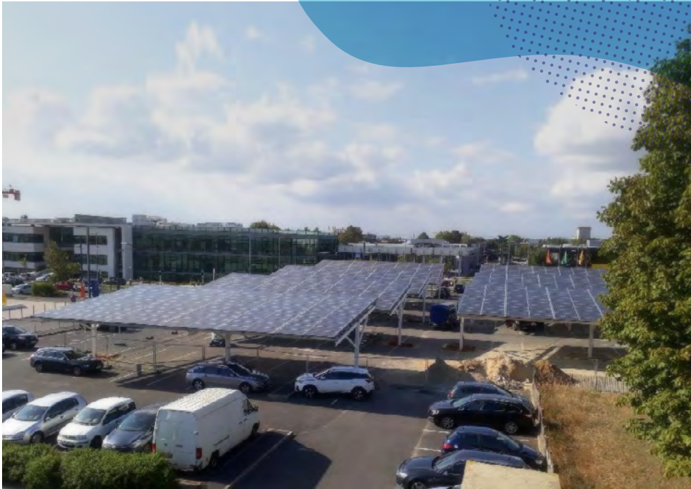
Photovoltaic shade structures, Paris-Orly-Rungis business park (Val-de-Marne)
