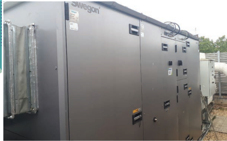
Photo: Heat pump
